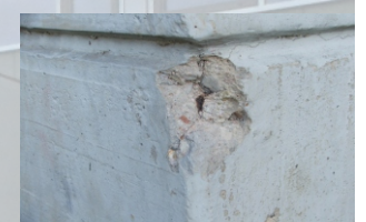
Damage pictures of concrete - Large area flaking due to reinforcement corrosion
